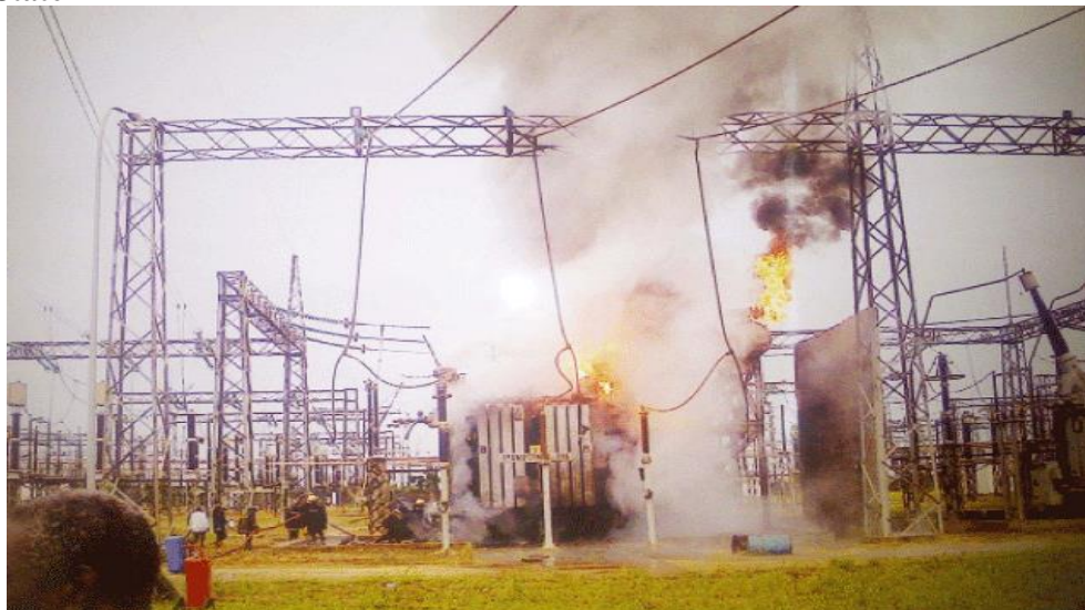
Figure 2: A typical overloaded electric power sub-transmission line, Alaoji, Abia State
